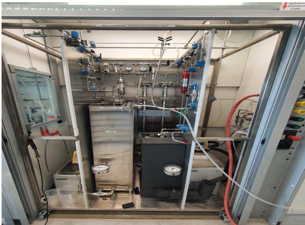
Fig-13. Butadiene Purification system
