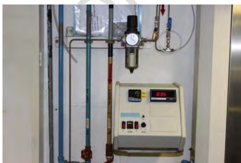
Fig-5. Reactor Controller
